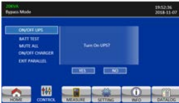
TURN ON UPS
