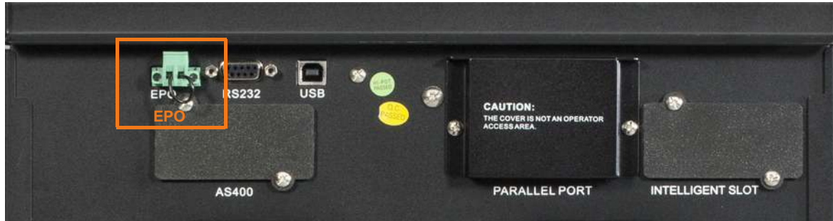
Figure 7.2 Emergency Power OFF
